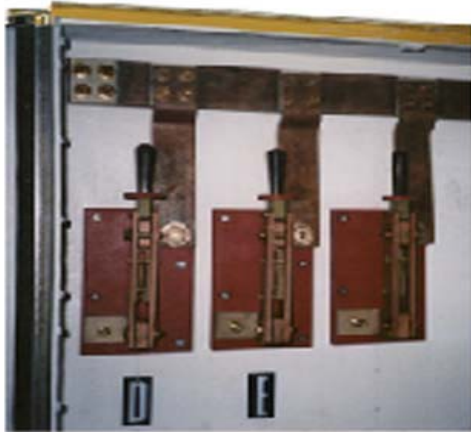
1200 AMP 750 VDC TRACTION POWER DISCONNECTS WITH SUPPLY BUS FOR CONNECTION TO ADJACENT SWITCH BOX
